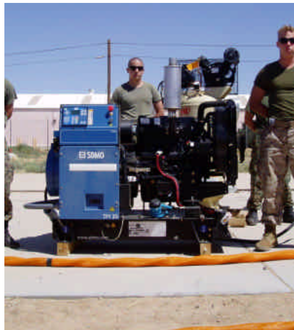
SDMO Diesel Generator X20
